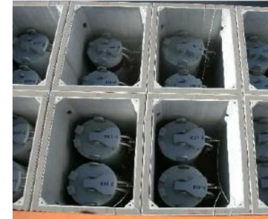
Temporary storage of the KURION adsorption towers
