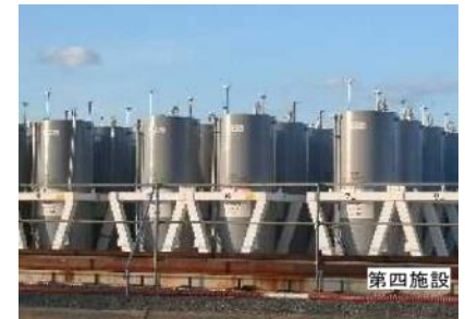
Storage of the SARRY adsorption towers
